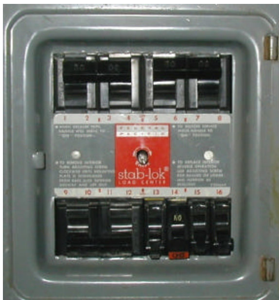
Figure 2 – Breakers that are on when down
