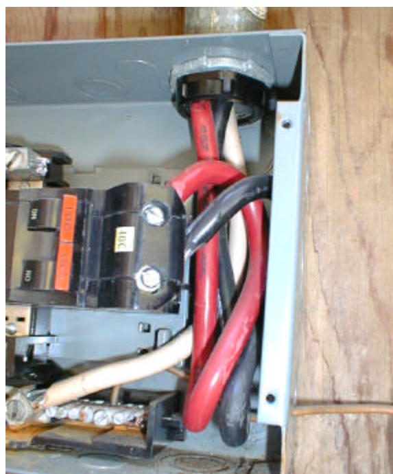
Figure 1 – Insufficient wire bending space
